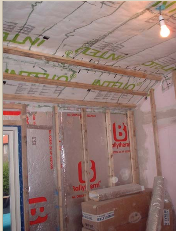
(left) Friction fit hemp wool insulation in the services zone; (below) dry-lining and air-tightness measures to improve the existing house
